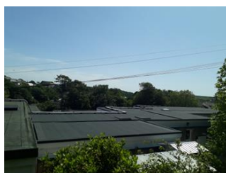
Parc Eglos School Full replacement of a significant section of flat roofing
